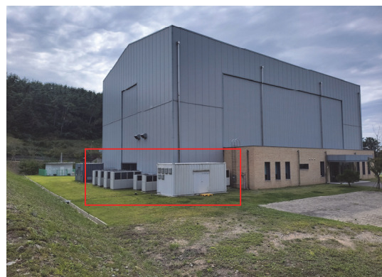
Fig. 2 Cold Room outside outdoor unit
