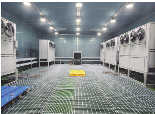
Fig. 1 Inside the Cold Room
