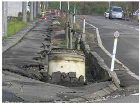
(b) Uplifted manhole and settled backfill (Konishi et al., 2008)
