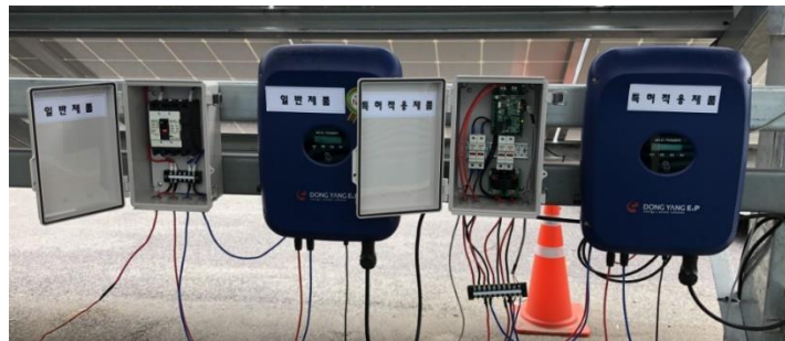
Figure 8. A Photo of the Installation of the Existing Connection Panel and the Connection Panel with the Digital Surge Detector
