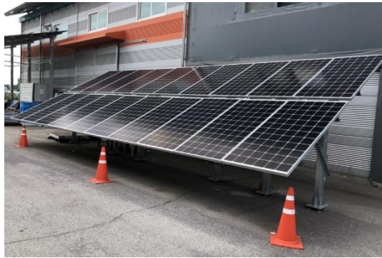
Figure 7. Field Pictures of Photovoltaic Module Arrays for Demonstration Experiments
