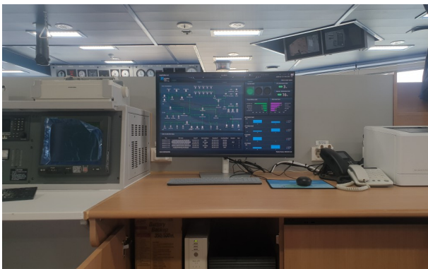
Fig. 8 SIEM installed on-board
