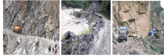
Fig. 2. Nepal's poor road infrastructures
