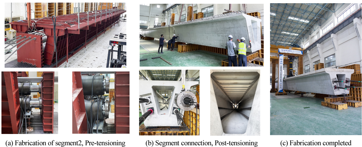
Fig. 4. Procedure of fabrication of PSC U shaped girder for the mockup test
