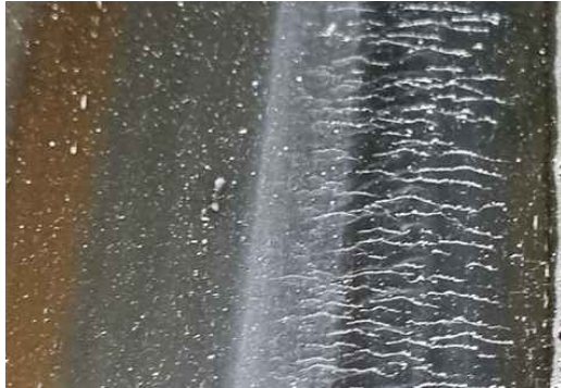
(a) Rail surface defects in braking section
