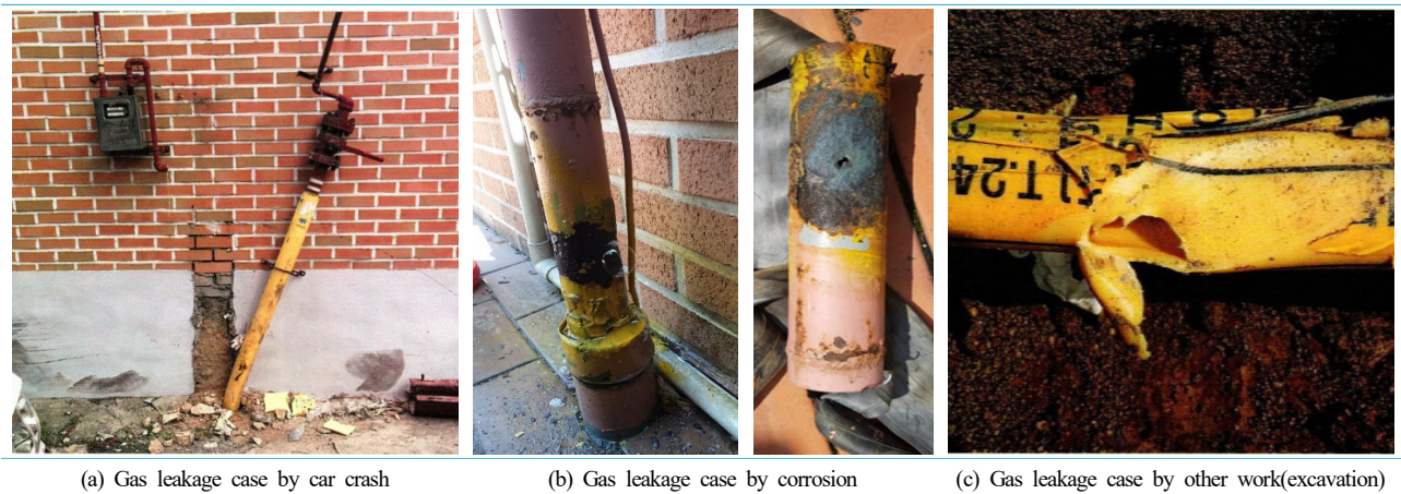
Fig. 1. The sample cases of gas leakage from pipe(including accessories).
