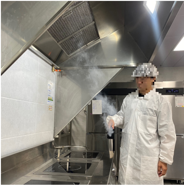
Figure 2. Photo of evaluating hood exhaust performance using smoke visualization
