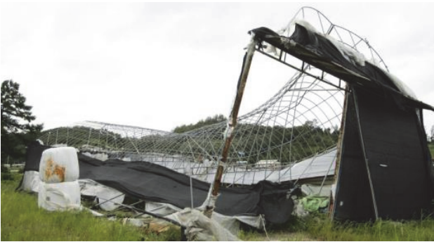
Fig. 1 Greenhouse damaged by wind load (RDA, 2012)
