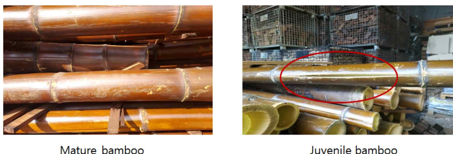
Fig. 10. V-shaped split and surface checks occurred in the longitudinal direction of the bamboo poles.
