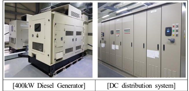
Fig. 2. DC distribution test bed composition equipment (Diesel generator & DC distribution system).
