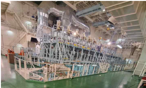
Fig. 6. Engine room in ship
