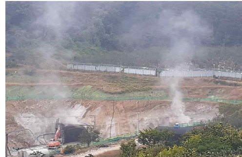
b) dust damage photo data at construction
