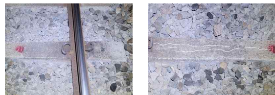
(c) Damage of concrete sleeper (#3)
