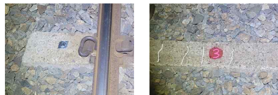
(b) Damage of concrete sleeper (#2)
