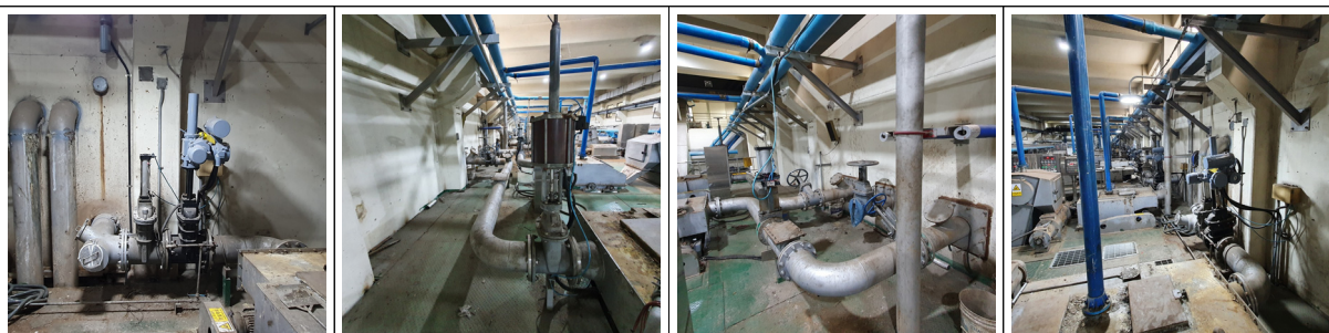
Fig. 2. Front piping and additional facilities of the Comprehensive treatment device for impurities.
