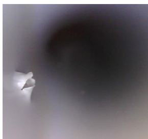
Figure 3. Defect photo in the pipe
