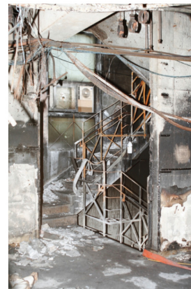
b) Main Stairwell after Fire 10)
