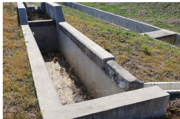
(b) Sand filter facility
