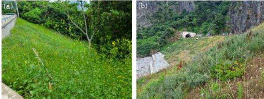
Figure 2. (a): Lapsana communis that grow densely between road and forest, (b): Intentional introduction of naturalized plants to road cutting sites in Ulleung-do.
