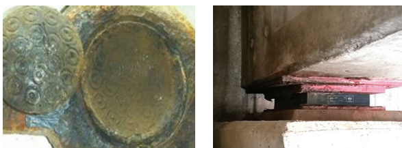
(a) high-strength brass friction material rust (b) corrosion of bearing supports due to rust
