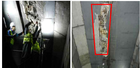
(a) Concrete cover lifting (b) Rebar exposed
