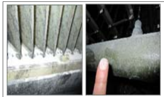
Fig. 4. FRP dust at the top of electrostatic precipitator.
