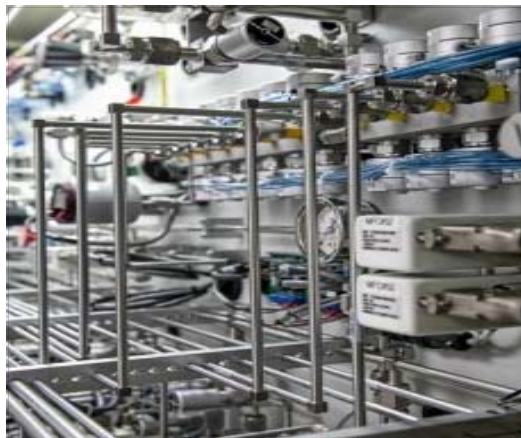
Fig. 1. ALD Gas Inlet Cabinet.
