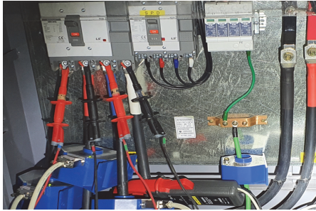
(a) Voltage measurement
