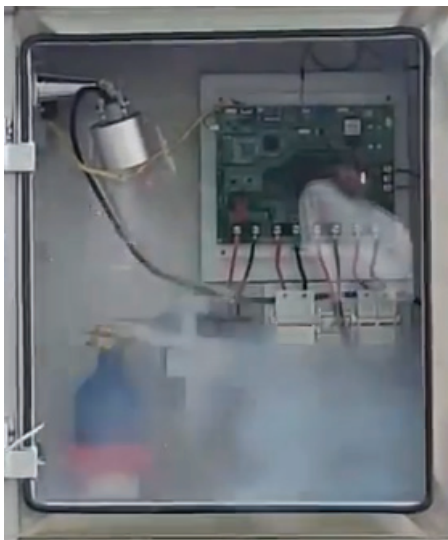
Fig. 8. Injection of fire extinguishing gas.
