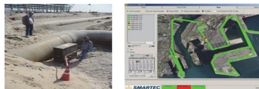
Fig. 6 SMARTEC : Pipeline Safety Monitoring Systems[22]
