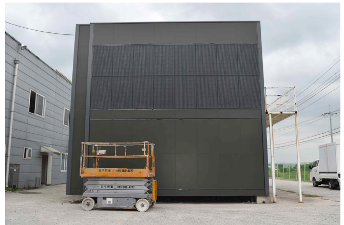
Figure 3. Examples of Wall Assemblies Mock-up : Pre-finished off-site factory manufactured wall (top), wall assembly mounted on two-story building (middle), wall assembly with BIPV attached (bottom)
