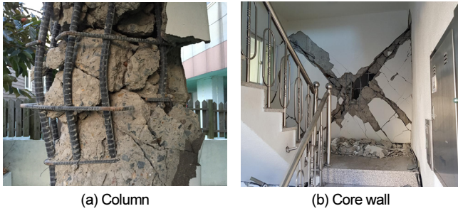
Fig. 1. Damage in piloti-type buildings at Pohang earthquake
