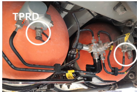
(b) Installed TPRD at the hydrogen tanks
