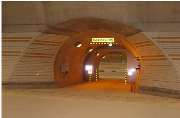
(a) General evacuation passageway in road tunnel
