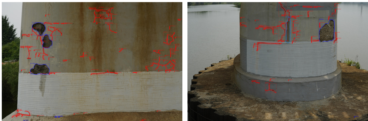
Fig. 7. Automatic damage analysis results in railway bridge testbed
