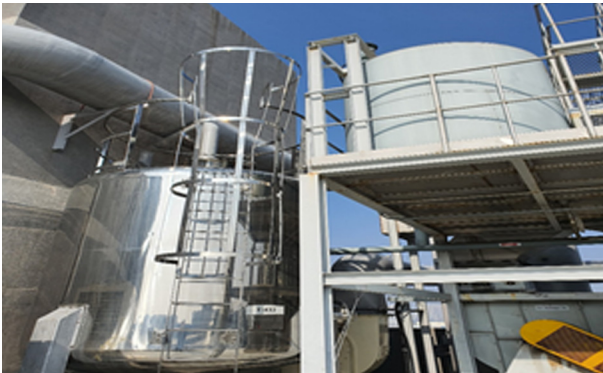
Fig. 11. Buffer tank system in the reaction process.
