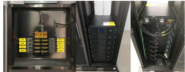
Fig. 8. Main power and UPS rack.
