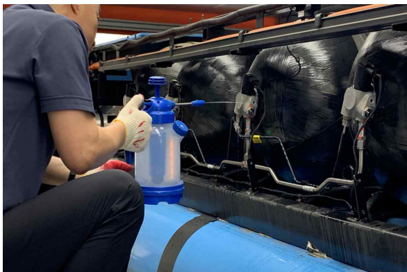
Fig. 2 Hydrogen leak inspection using a bubble
