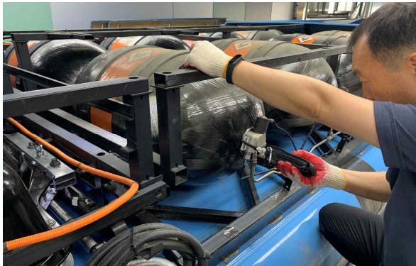
Fig. 1 Hydrogen leak inspection using a hydrogen detector
