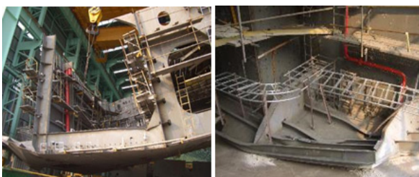
(a) Damaged blocks
