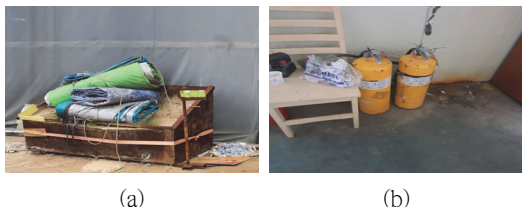
Fig. 1 Dry sand (a) and class D fire extinguishers (b) in magnesium recycling factory
