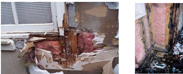
Fig. 1. Cases of Defects in Lightweight Wooden Structure Walls with External Thermal Insulation Composite Systems 12)
