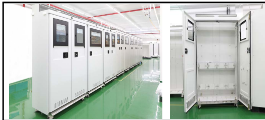
Fig. 3. General appearance of gas cabinet.
