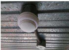
(c) By moisture in places outside the parking lot
