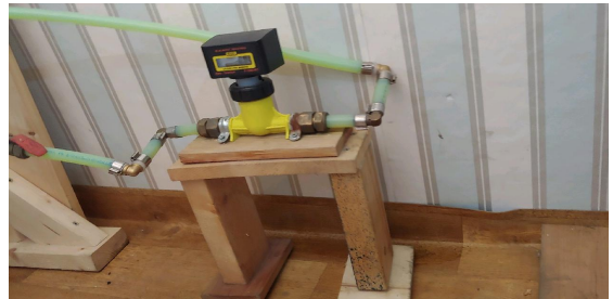
Fig. 4 Ocher jjimjilbang hot water flow measuring device
