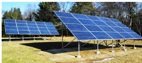
Fig. 2. Ground mounted solar PV 51)
