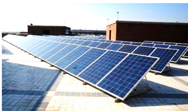
Fig. 3. Roof top solar power PV plant 52)
