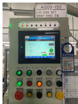
(a) Control Display Using Push Button and Touch Screen.
