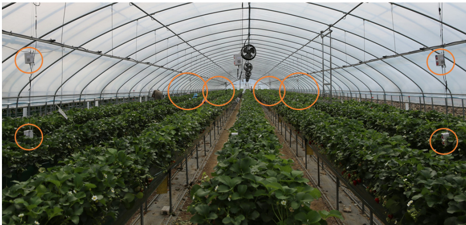
Fig. 2. Picture of installed sensor nodes in the experimental facility.
