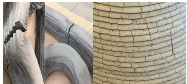
Fig. 1 Shrinkage crack on 3D printed layers (Jo et al., 2020; Moelich et al., 2020)
