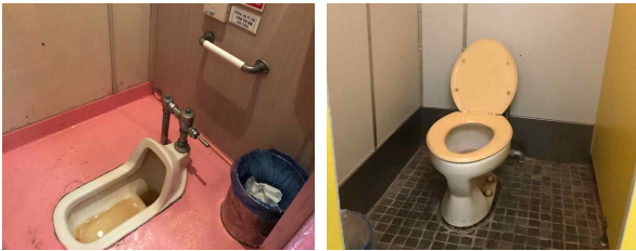
Fig. 1 Older toilets of women's restroom
