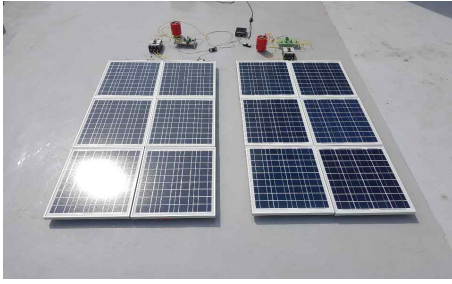
Fig. 8. Experimental environment for PV generation (3Sx2P Connection Structure).
