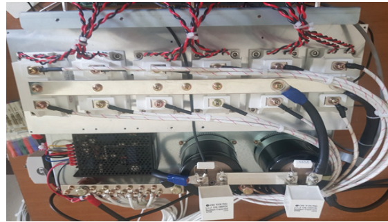
(b) Power Stack
