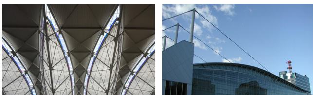
(a) Web Rod of Truss in San Francisco Airport (b) Tension Cable in Makuhari Messe
