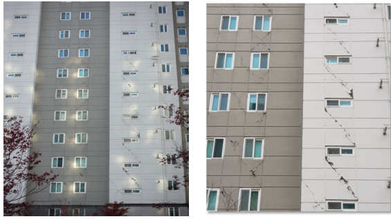
〈Fig. 1〉 Pohang S apartment damage after earthquake
